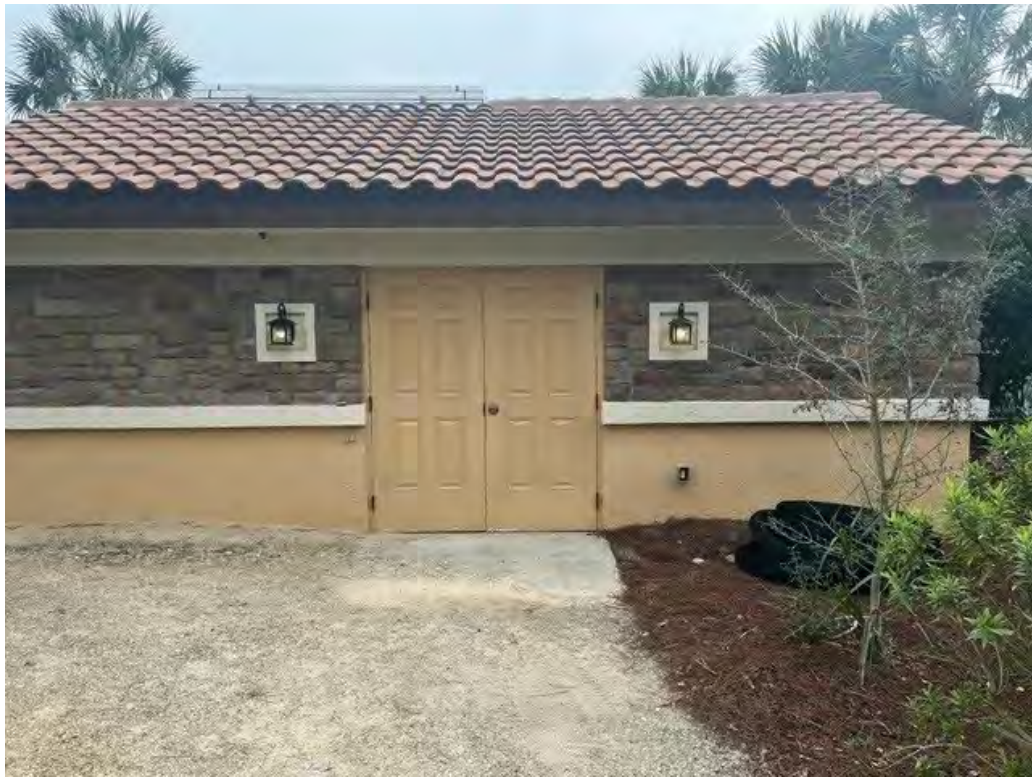
Irrigation - Pump House (External)
