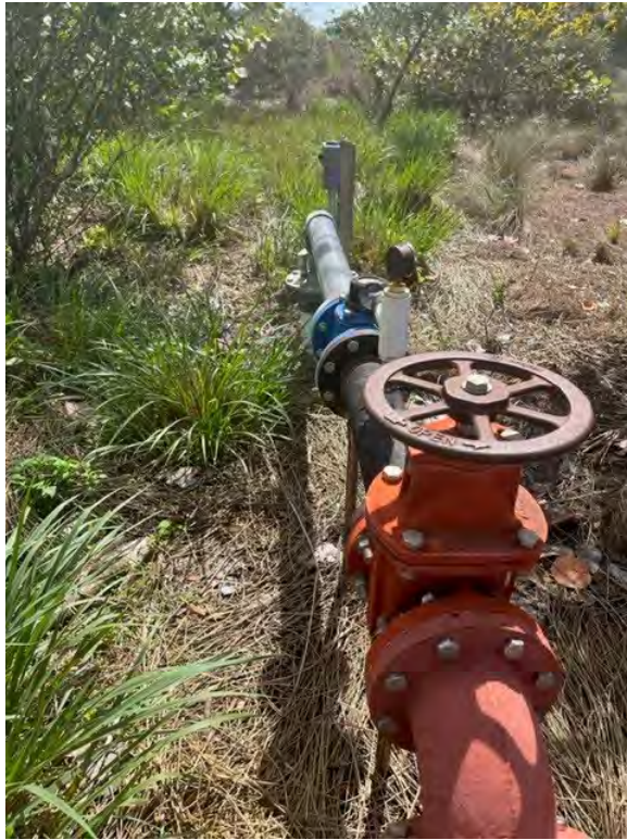
Irrigation - Recharge Well - Hole 11
