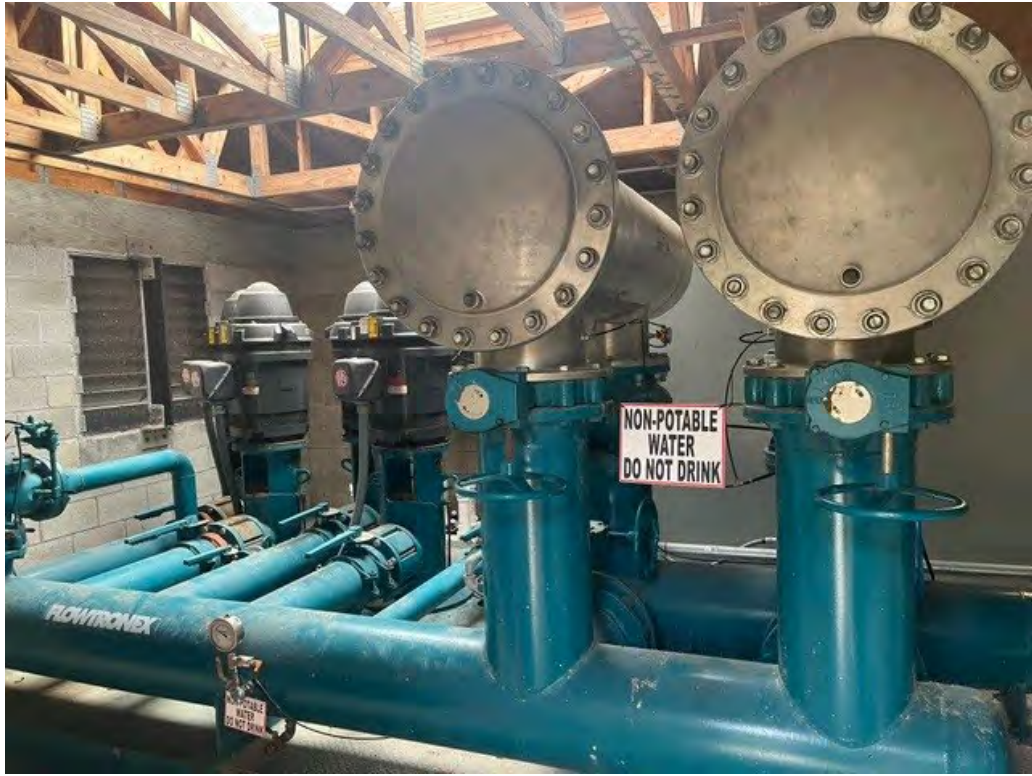
Irrigation - Pump House (Internal)
