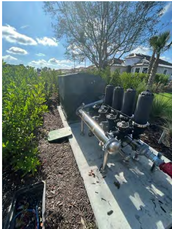
Irrigation - Pumps - Hatcher Parcel
