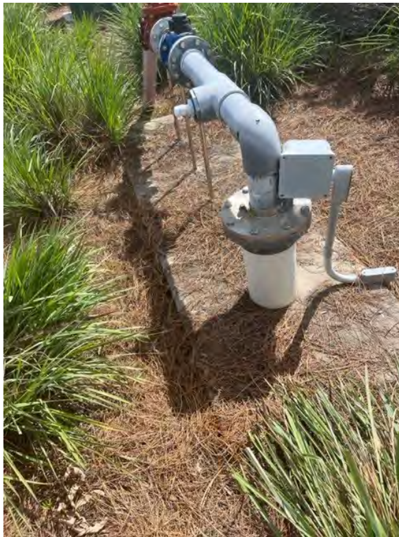
Irrigation - Recharge Well - Hole 12
